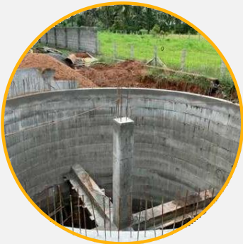
Underground Water Tank
